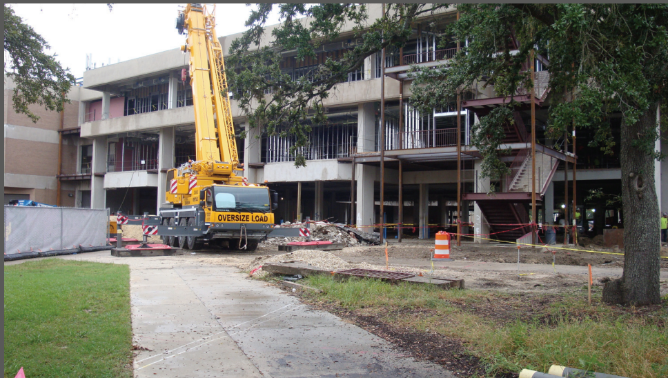
The first floor will house food services, the second will feature research lab space, and the third will have mechanical engineering faculty offices.
